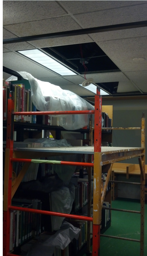
Pictures of Water Leaking on Expensive Art Books
