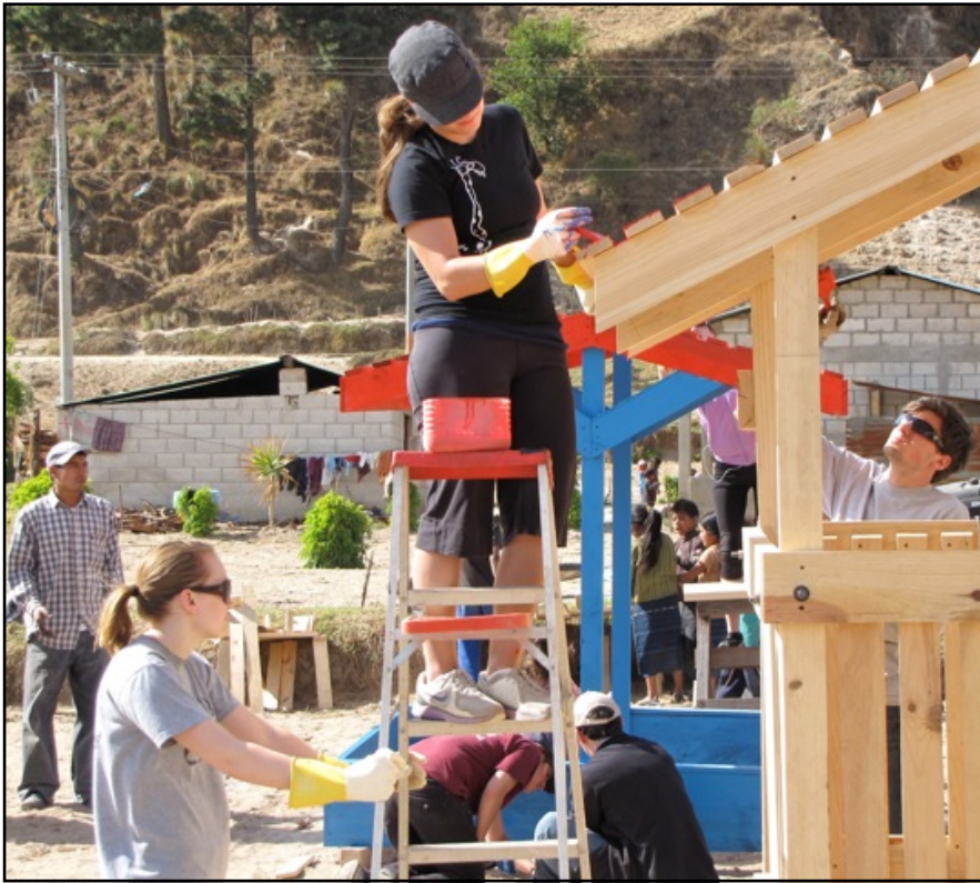
Ramapo students building a covered playground during their Alternative Spring Break in Guatemala
