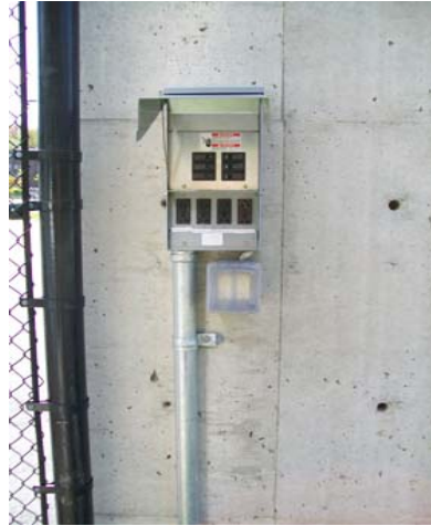
6- 120 Volt 20 Ampere Circuits Each Duplex receptacle is a circuit
