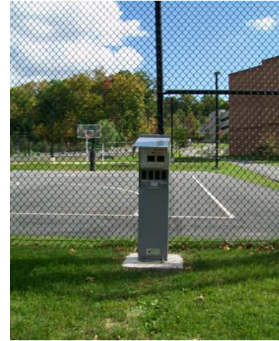
4-120 Volt 20 Ampere Circuits Each Duplex receptacle is a circuit
