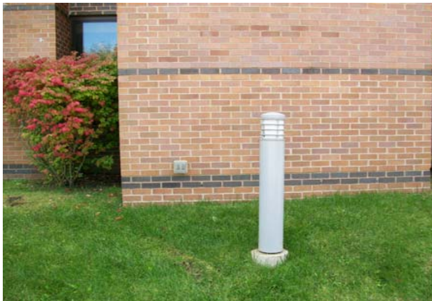
2- 120 Volt 20 Ampere Circuits Each Duplex receptacle is a Circuit
